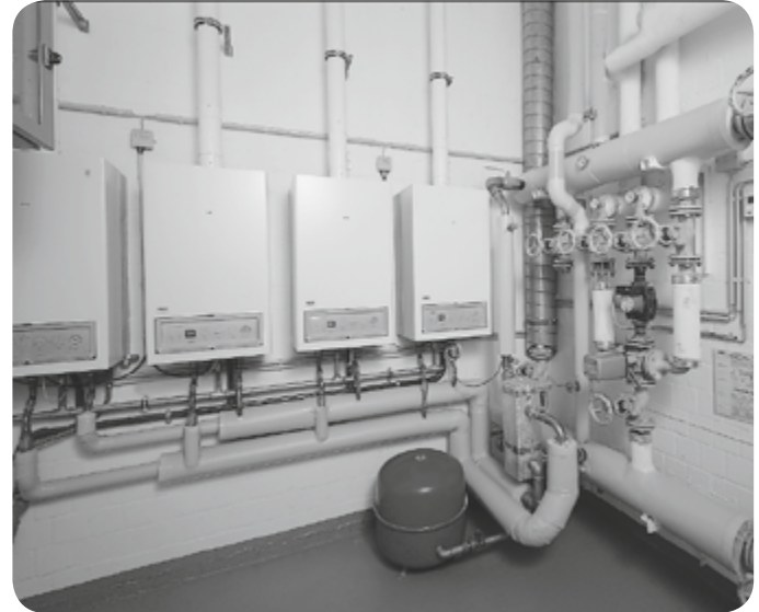
Heating boilers connected in cascade
